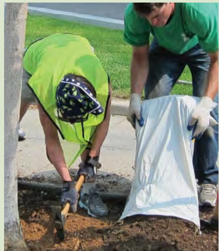
Fig. 36 After weeding the box around a city tree, we spread a thin layer of mulch.
